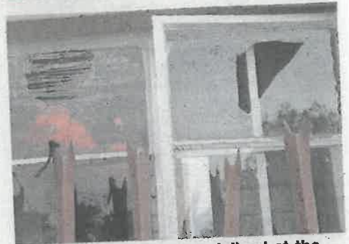
The guard room was vandalised at the Department of Basic Education in Letlhabile. Photo by Samson Ratswana
